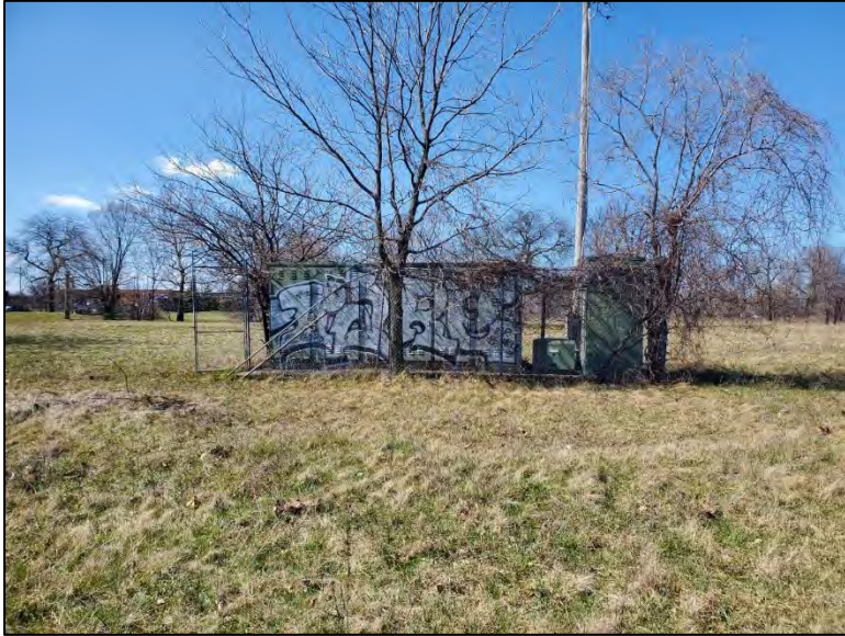
Photo 33: Electrical transforms within Project Area, facing northeast.
